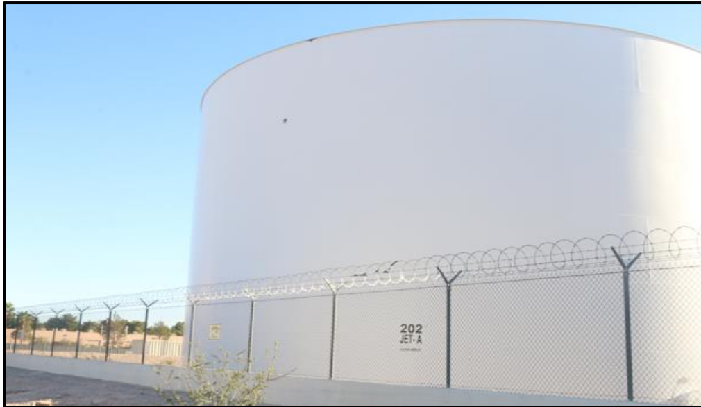
(McCarran International Airport fuel tank with bullet strikes.)
