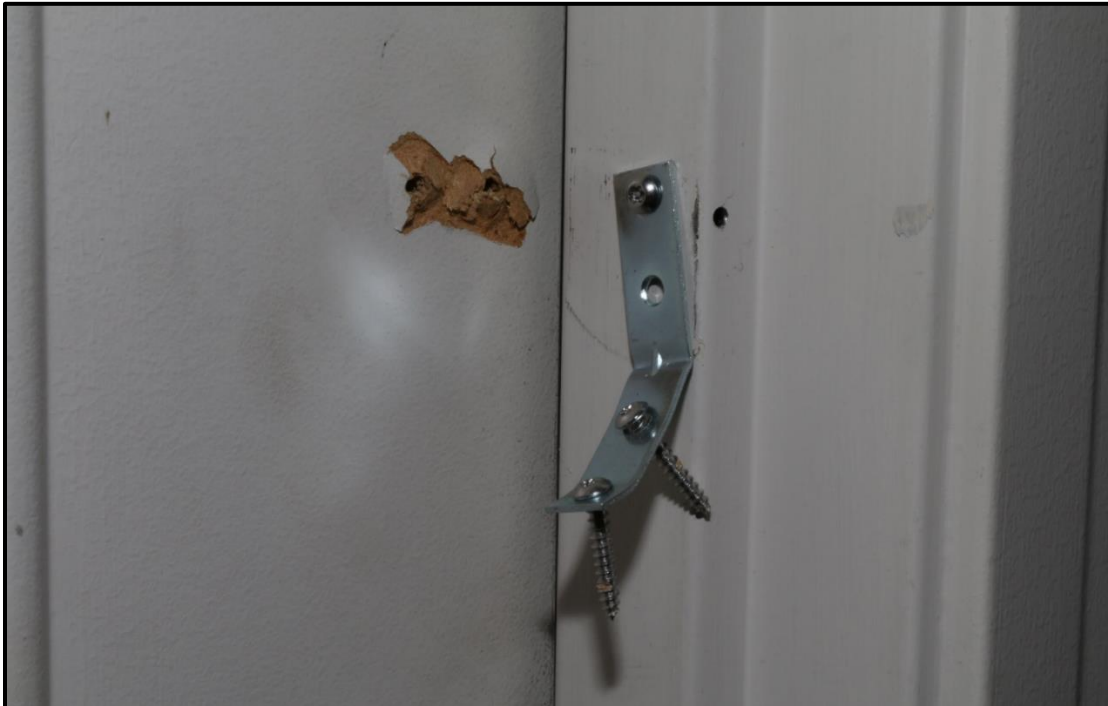
("L" bracket after the door was manually breached.)
